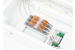
Multi-pole, fixed lighting fixture wiring
